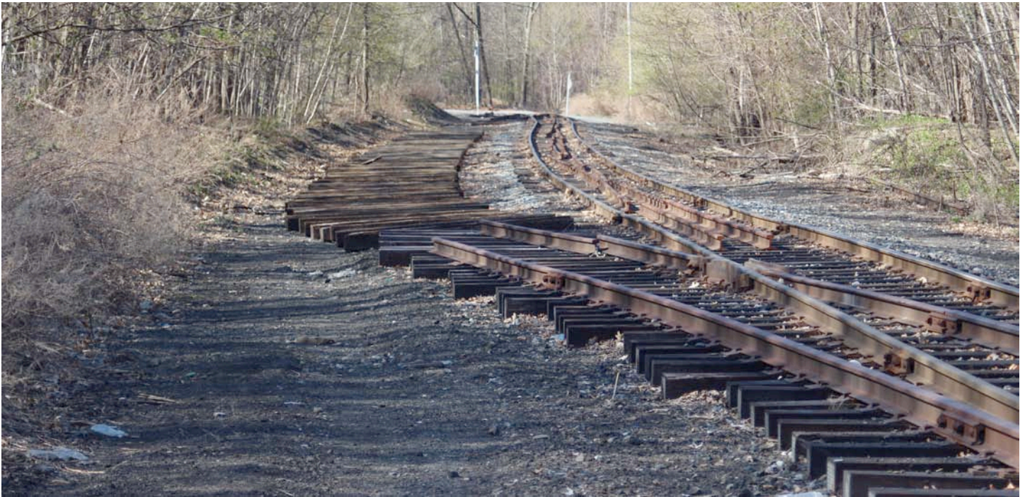
By April 18 th , the M&NJ resumed construction of a runaround between Houston Ave. and Washington St., on the south side of DG yard. Randy Stone's photo looks toward Washington St. Rail sections lie within the main line's gauge.
